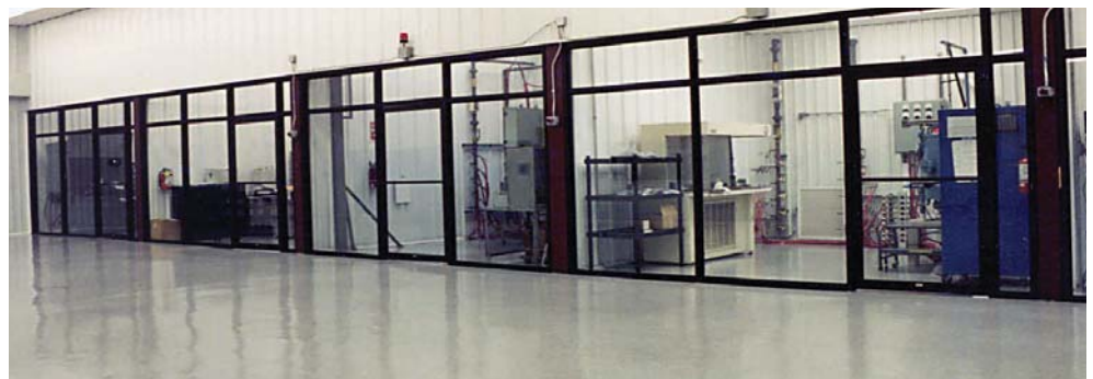
Individual bays for each CVD SiC reactor fitted with dedicated HEPA-filtration system.
