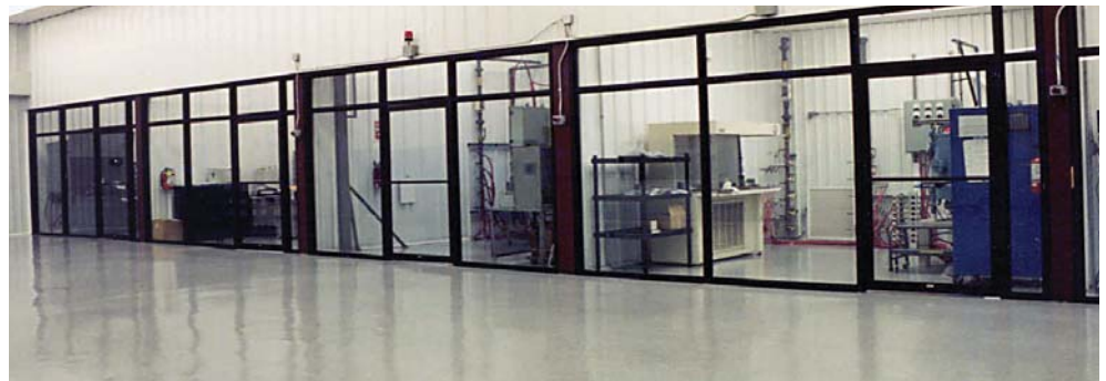
Individual bays for each CVD SiC reactor fitted with dedicated HEPA-filtration system.
