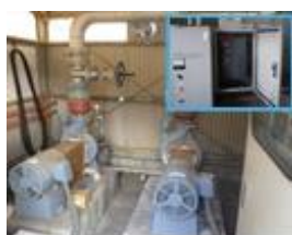
Inverters of circulation pumps (after) Case 1 (Hadano Facility)
