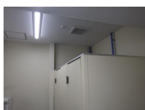
LED lamp with motion sensor (after) Case 3 (Oguni Facility)
