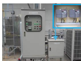
Inverters of cooling water pumps (after) Case 4 (Nagasaki Facility)
